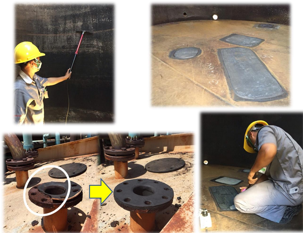
Upper left: Pinhole test, Upper right: Bottom plate repair completed Lower left: Defect on piping flange part restored, Lower right: Repair work for bottom plate
